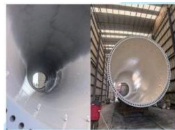
Guangxi Wind Power Project
